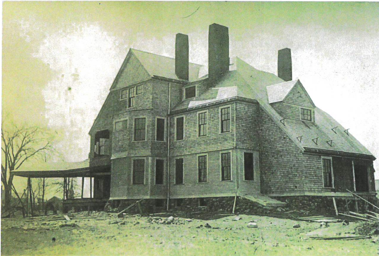
The Van Kleeck mansion, known as Rock Lawn, under construction in the late 1880s.
