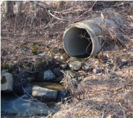
Figure 1: Drainage pipes transport stormwater to local rivers and ponds, including the Bogastow Brook and the Charles River.
