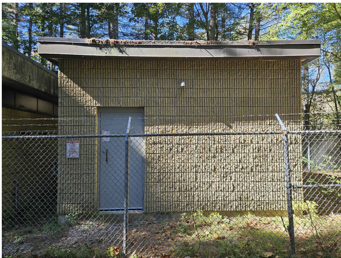
7. EAST SIDE OF PIPING BETWEEN CHEMICAL FEED BUILDING AND WELL PUMP HOUSE FACING WEST
