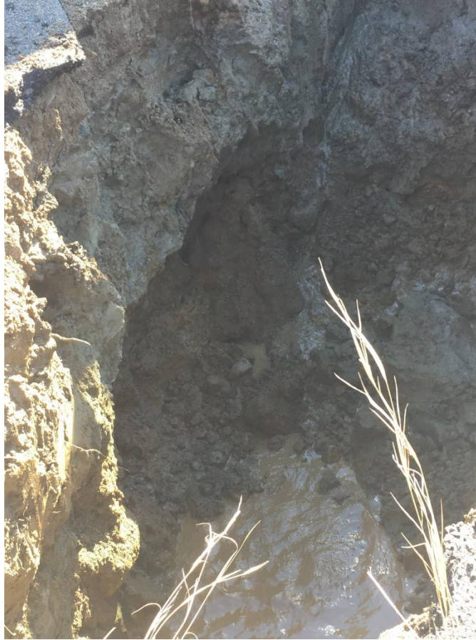
Infil-200 Testpit, water weeping into test pit at 20"
